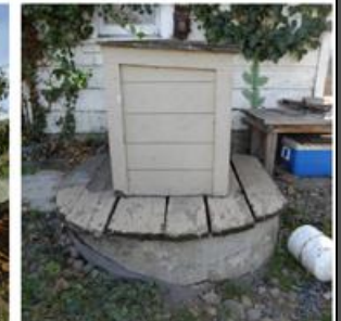
Image 3 - Pump house on the Rodrigues Farmhouse Property, taken from the southeast
