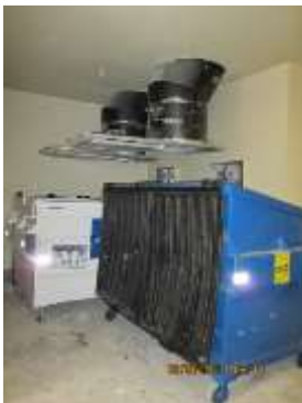
Figure 3: Garbage and recycling chutes
