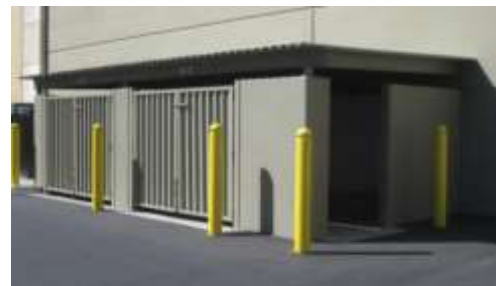
Figure 15: Personnel door on enclosure
