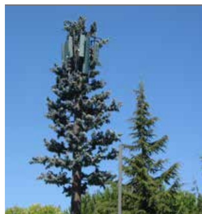
The above two faux trees have exposed antennas with no covers or needle socks and insufficient foliage and branches to hide equipment.
